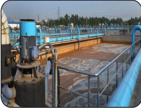
EFFLUENT TREATMENT PLANT
