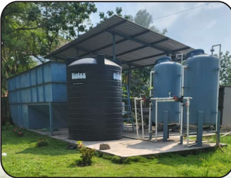
SEWAGE TREATMENT PLANT
