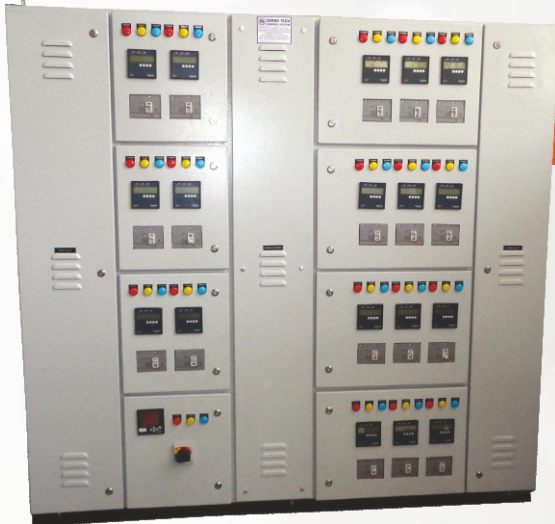
HOUSE METERING LIGHTING PANEL
